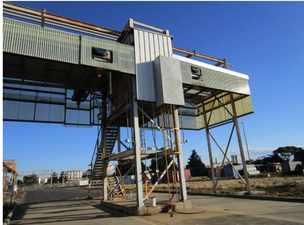
Figure C13.1 Dow's tanker truck loading station – this facility will be rebuilt for loading out Plasticrude and Heavy Fraction oils.
