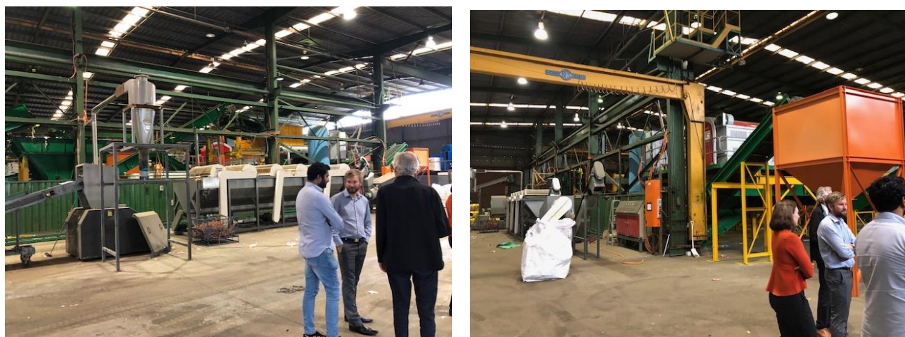
Fig C4.1 Pics of iQRenew’s Tuggerah Plastics Preparation facility
