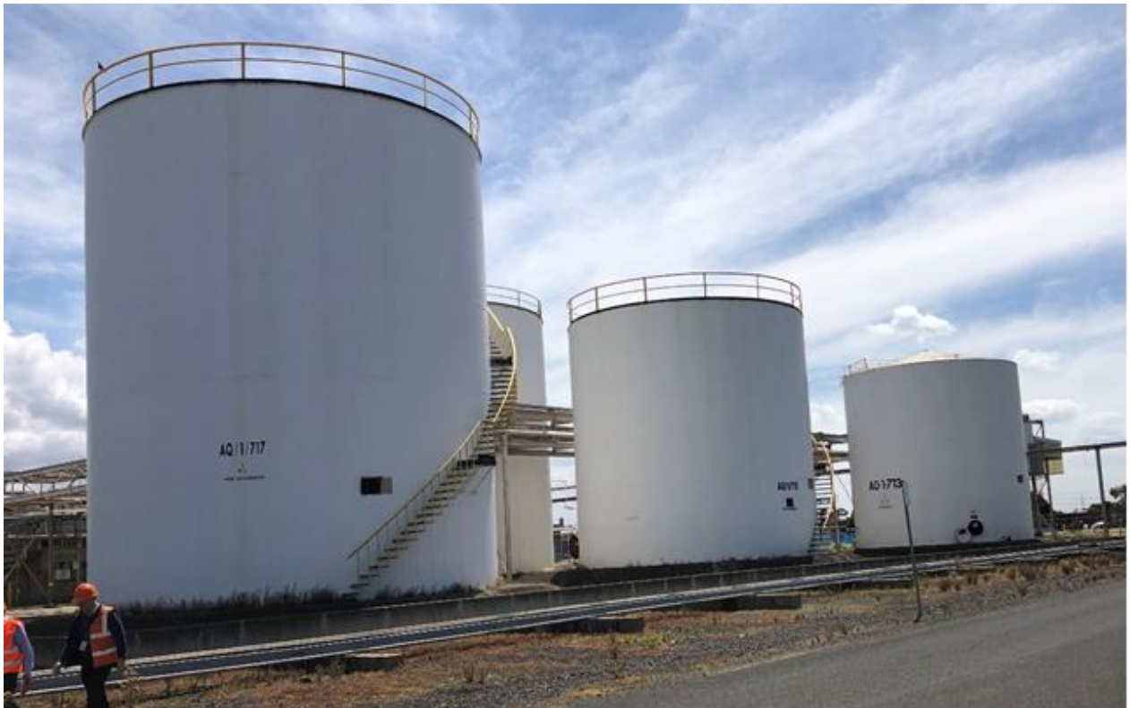
Figure C12.1 Product tanks at the Altona Dow site that are available for refurbishing into Plasticrude Product tanks for the Advanced Recycling facility
