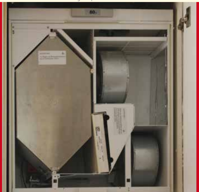
Ventilation unit with heat exchanger exposed.
