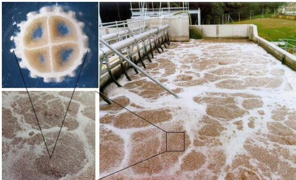
Figure 2. Full-scale Moving Media wastewater treatment plant for a municipality.
