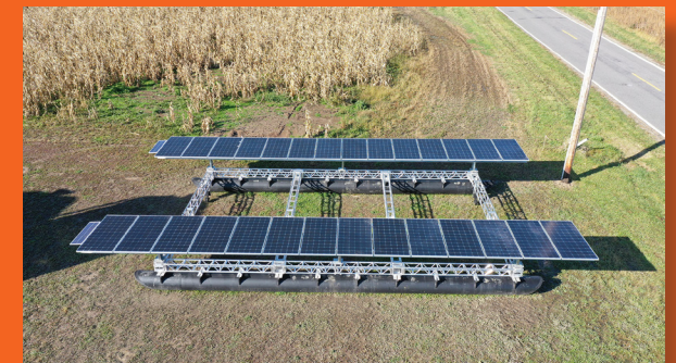
A 11.2kW TrackerSled pilot operating at Granor Farm, Three Oaks, Michigan
