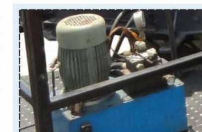
HYDRAULIC POWER PACK
