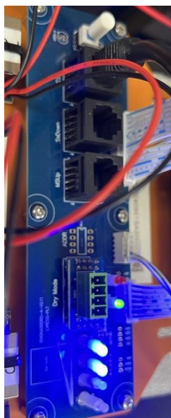
Blue and Green Lights on the Communication Adapter Board Indication the BMS is Turned-On
