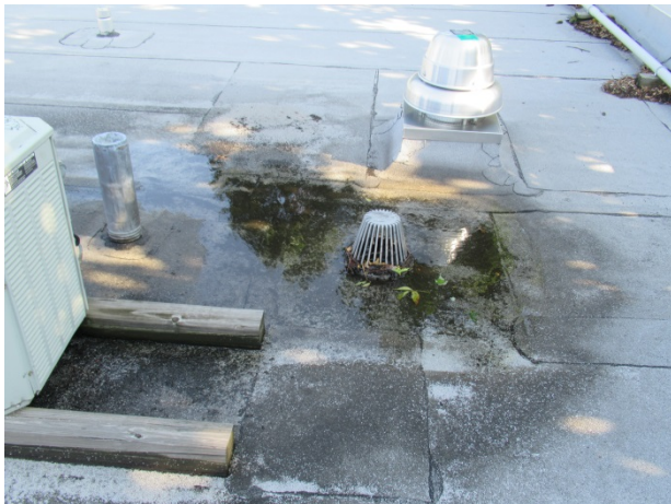
Ponding water and build-up at drain
