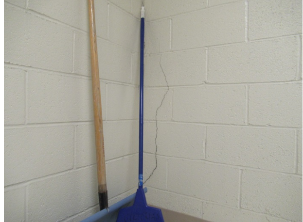
Masonry wall and finish crack
