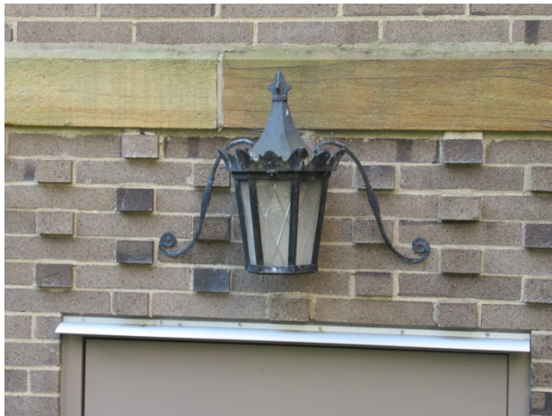
Exterior light fixture, note finish deterioration
