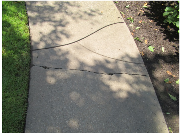
Rear courtyard crack
