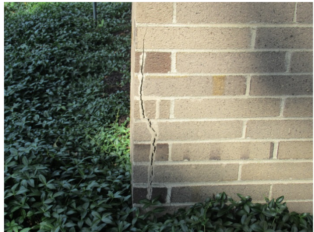
Masonry cracks and previous repair
