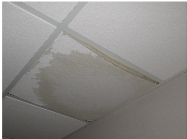
Stained hallway acoustical ceiling tiles, located near Unit 205
