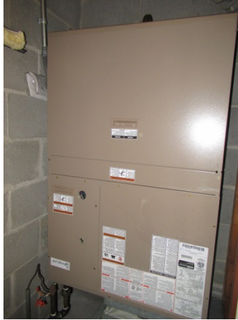
Split system furnace
