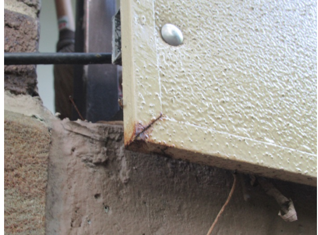
Minor panel rust
