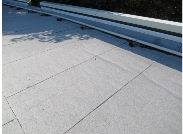
Isolated loose membrane
