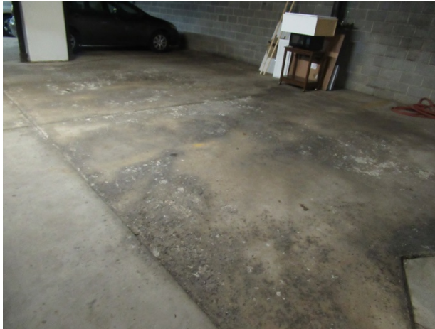
Spalled on-grade concrete
