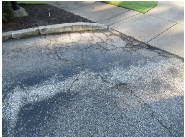
Front pavement cracks and settlement
