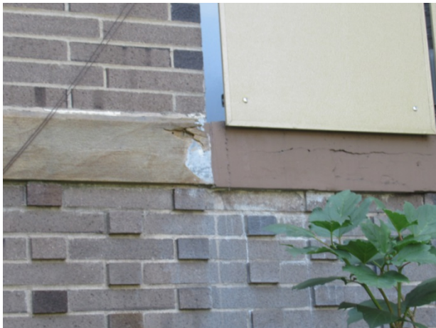
Damaged stone masonry and repairs
