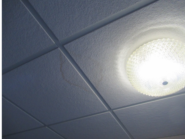
Ceiling tile stain at hallway
