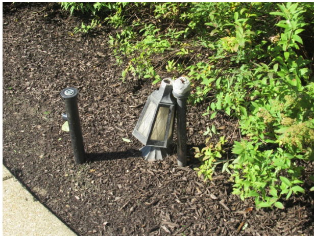
Bollard in poor condition
