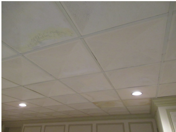
Stained ceiling tiles
