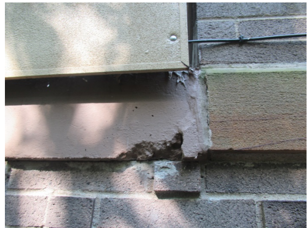
Spalled balcony concrete
