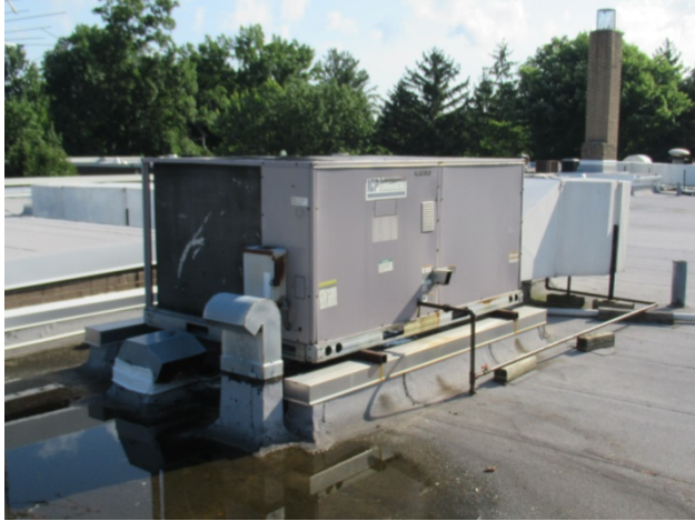
West hall rooftop unit
