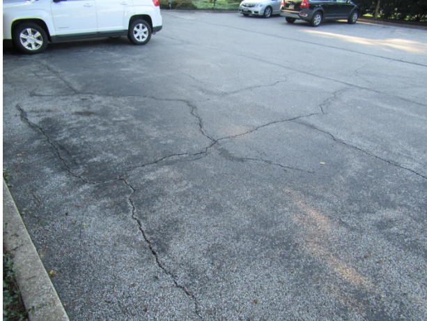
Front pavement cracks
