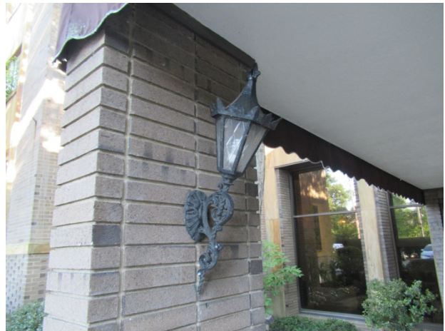
Exterior light fixture, note finish deterioration
