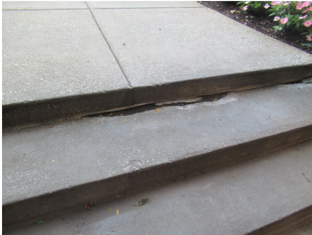
Entrance concrete step deterioration
