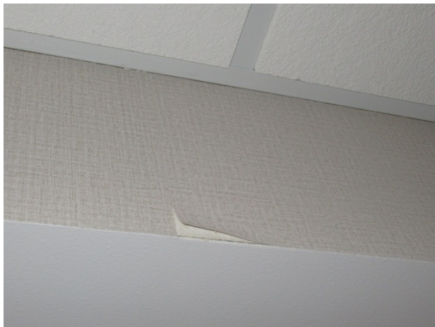
Lifted wall coverings
