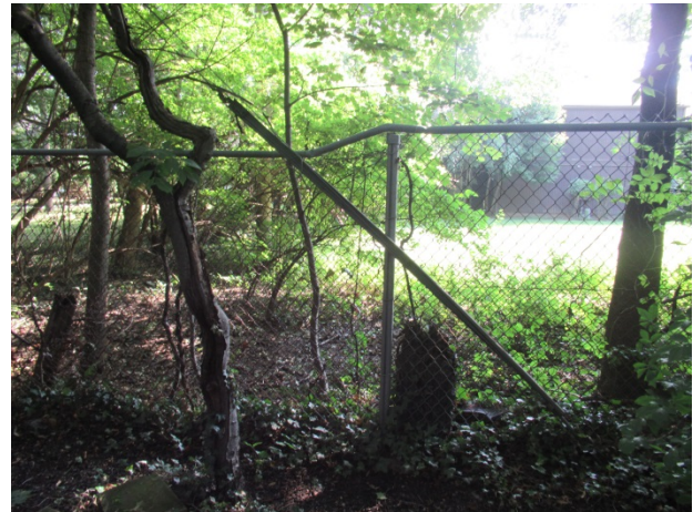
Damaged section of chain-link fence
