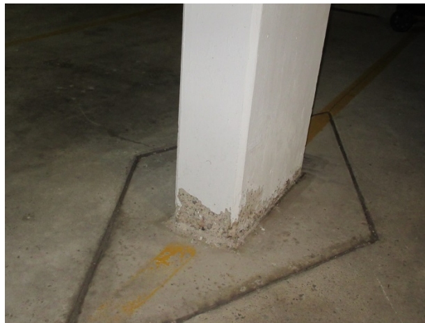
Spalled concrete column
