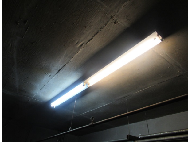
Garage light fixture
