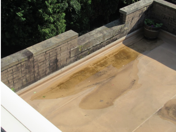
Loose membrane and ponding water at balcony
