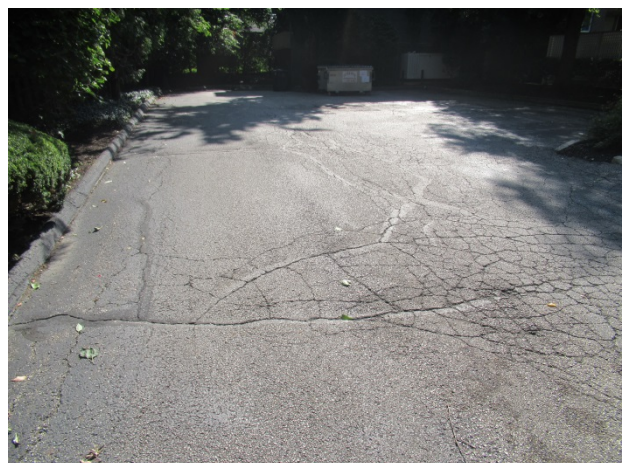
Rear pavement alligator cracks
