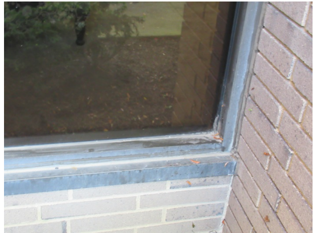
Lobby window frame, note discoloration
