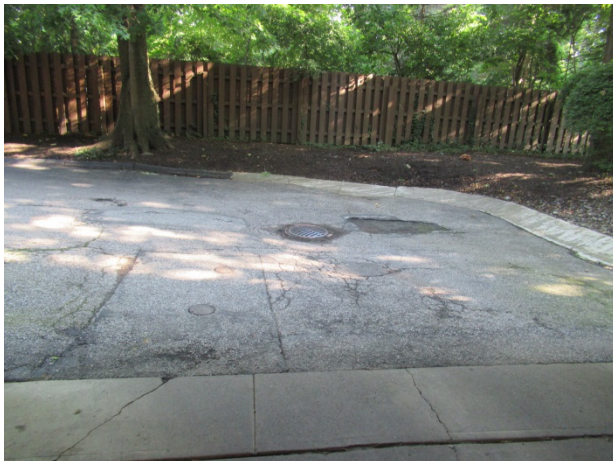
Rear pavement potholes and deterioration
