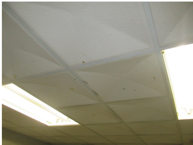
Damaged ceiling tiles in billiards room
