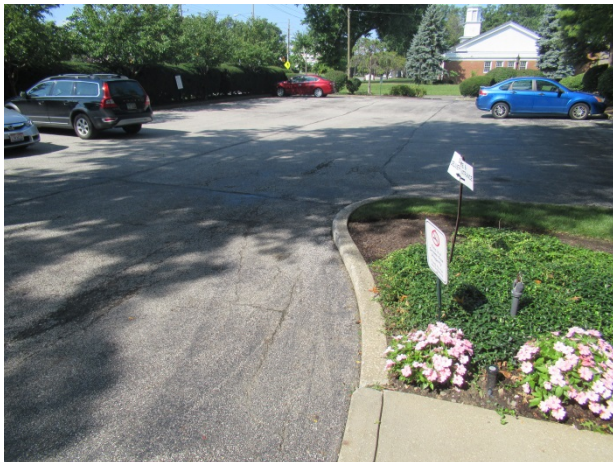
Front parking area pavement
