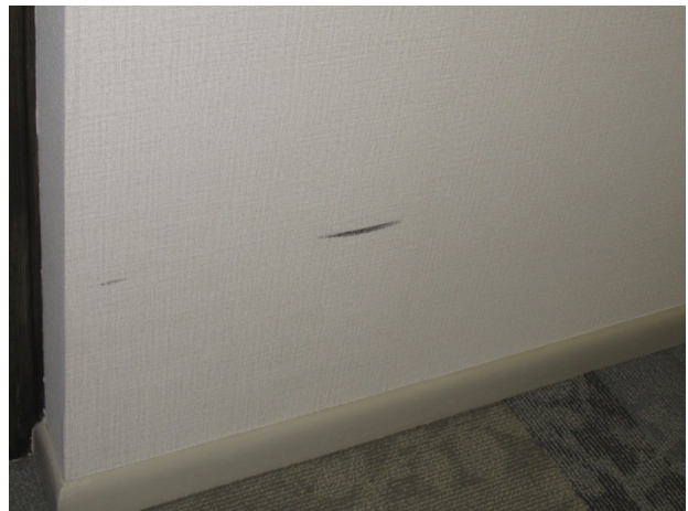
Scuffed wall coverings
