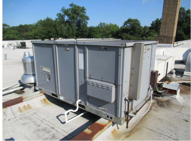
East hall rooftop unit
