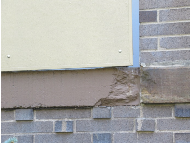
Spalled balcony concrete
