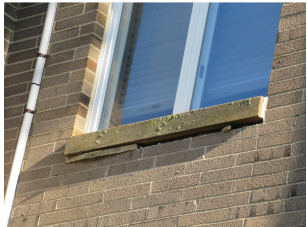
Mortar loss below window sill
