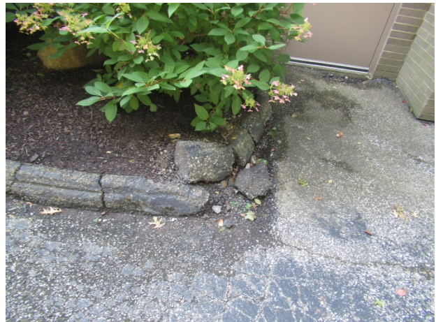
Rear pavement and curb deterioration
