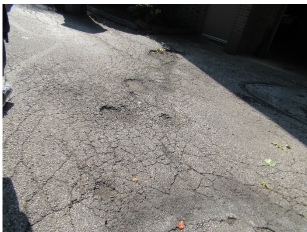
Rear pavement potholes, cracks and deterioration
