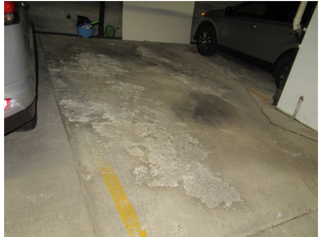
Spalled on-grade concrete
