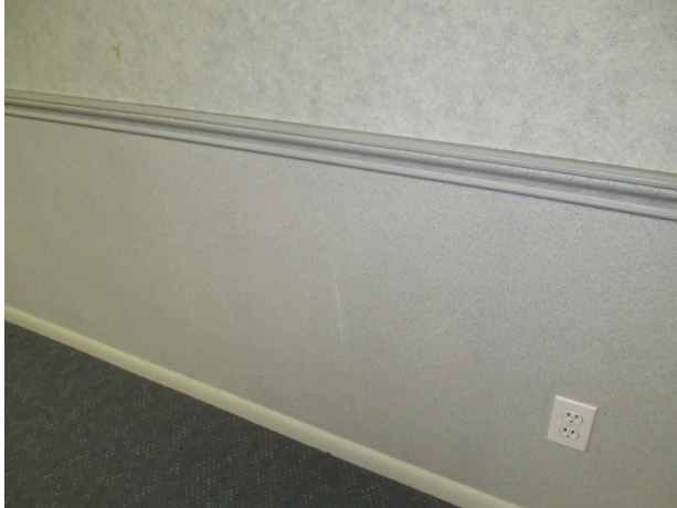
Scuffed wall coverings at billiards room
