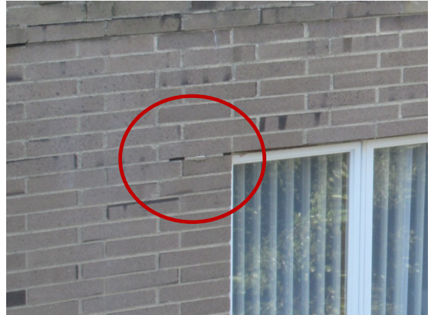
Mortar loss at lintel
