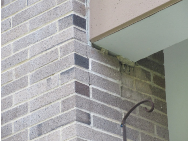
Cracked and spalled masonry below balcony
