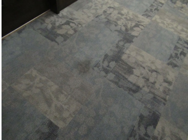
Hallway carpet stain
