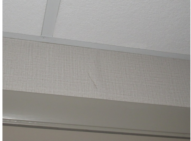
Torn wall coverings at second floor
