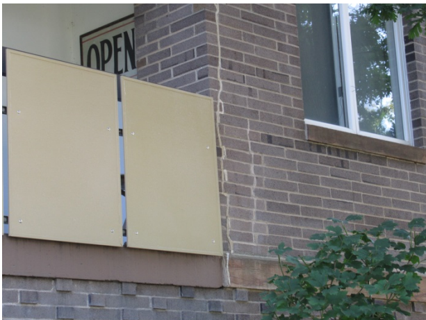
Previous masonry repairs
