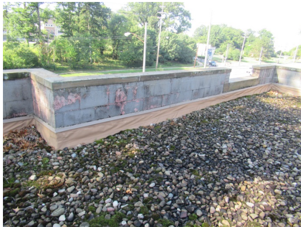
Loose membrane at built-up roof section
