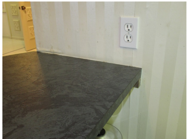
Loose wall paper
