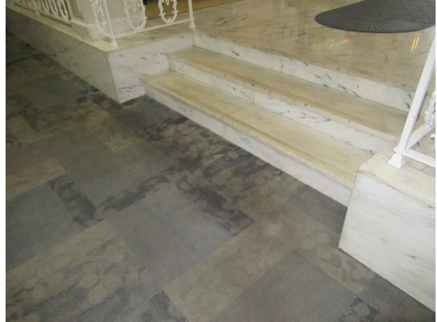
Carpet discoloration near lobby
