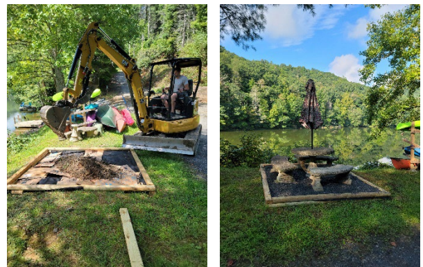
Chris Roten (VP) working on the new bench area and finished product.
