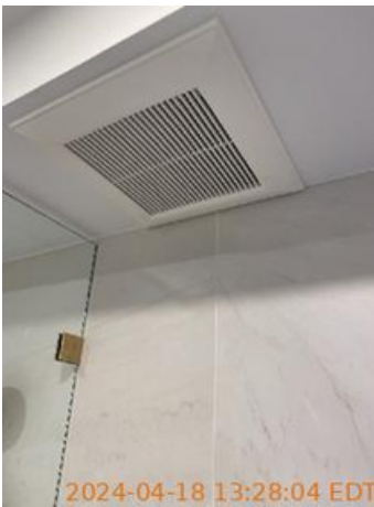
Exhaust Fan □ 2024-04-18 13:28:04 □ 25.82951194211311, - 80.12079559072873 □ Image
