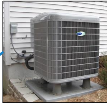
Outdoor Unit - looks like central AC
