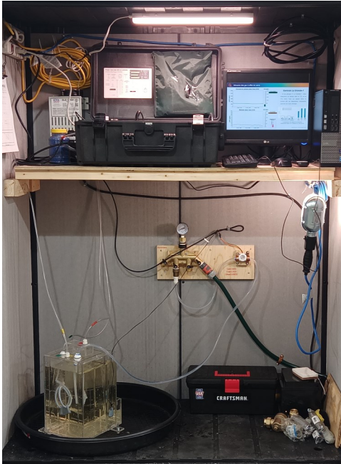
Installation in generating station in line with the SAGES
