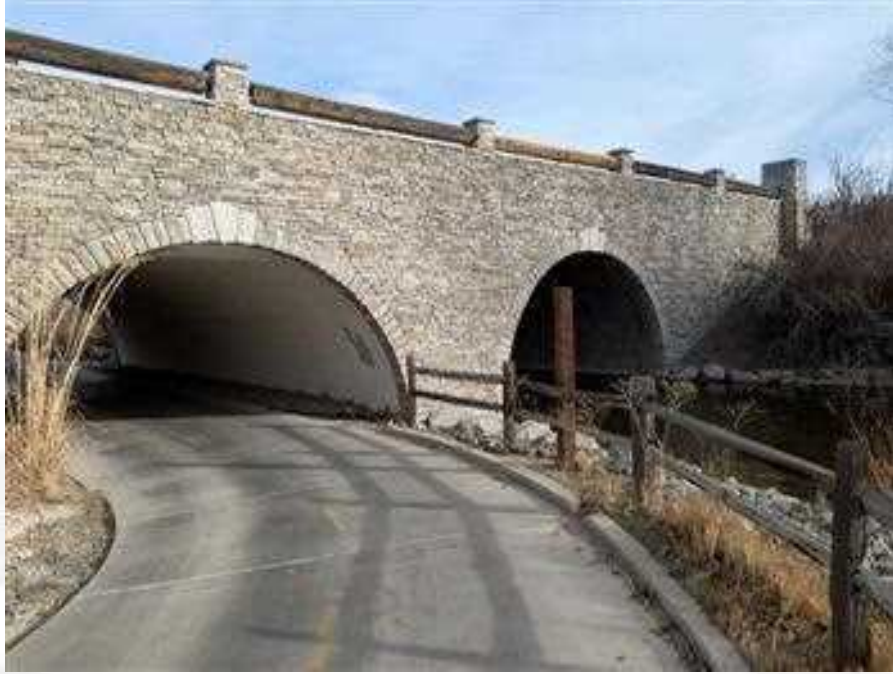
2 cell 20' diameter Arch Culverts, North Truckee Drain under Wingfield Springs Road/Silverton Way
