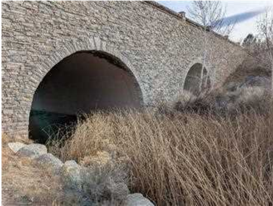
2 cell 20' dia Arch Culverts under Wingfield Springs Rd near Cinnamon Dr.
