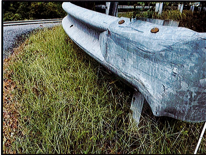
Figure 6: Damaged Guide Rail
