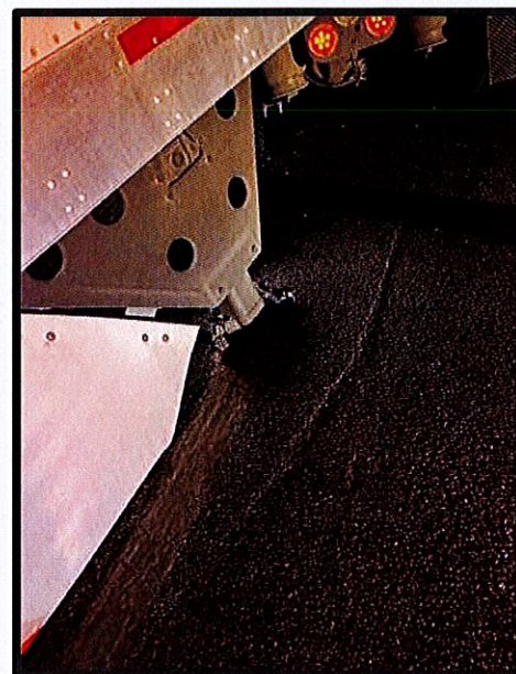
Figure 3: Pavement Damage from Truck
