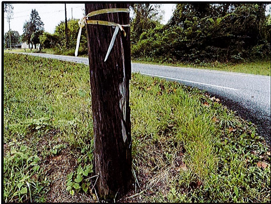
Figure 8: Damaged Utility Pole Shady Lane and Old Trail Road
