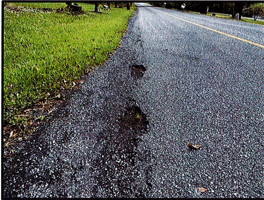
Figure 7: Pavement Distress on Shady Lane
