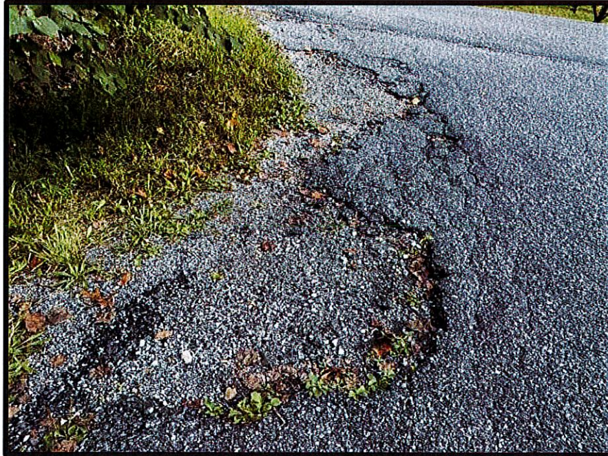
Figure 4: Shoulder Deterioration on River Road
