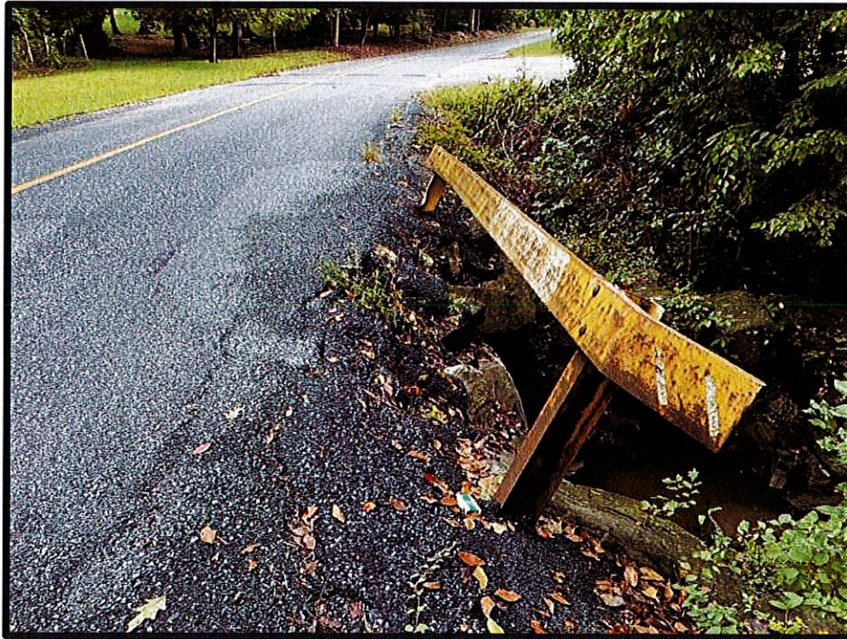
Figure 11: Shady Lane Roadside Hazard
