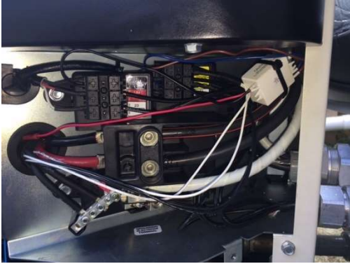
Figure 14 - Inverter secured with zip tie
