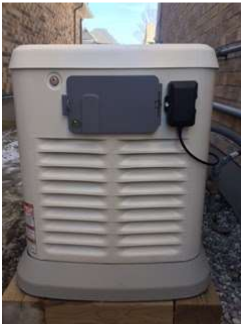
Figure 5 - Monitoring device mounted on generator
