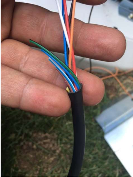
Figure 7 - Unused wires clipped
