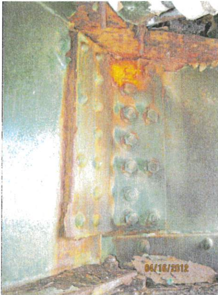
Deterioration of the Beams and Connections
