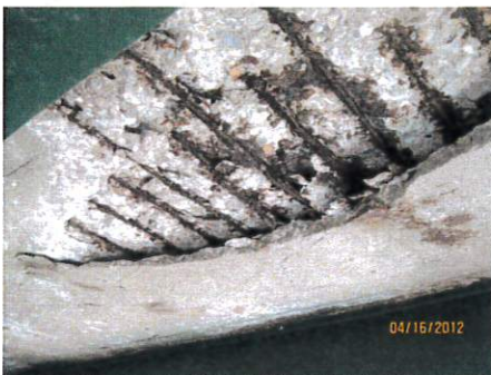
Exposed Rebar Underneath the Bridge Deck
