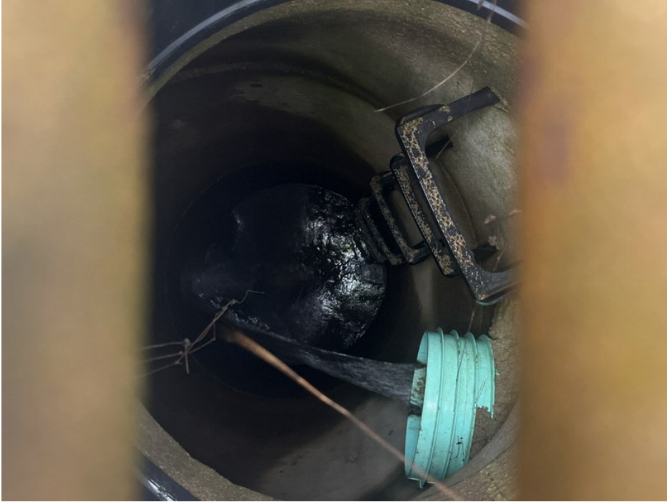
View inside outlet structure. Remove debris.
