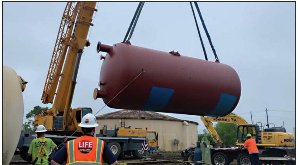
Last fall, two of the city’s eight water filter vessels were replaced.
