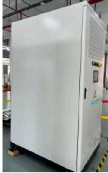
Energy Storage System (Left view)
