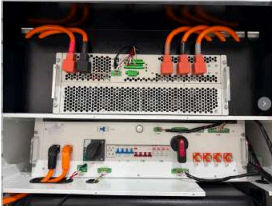
Battery control box
