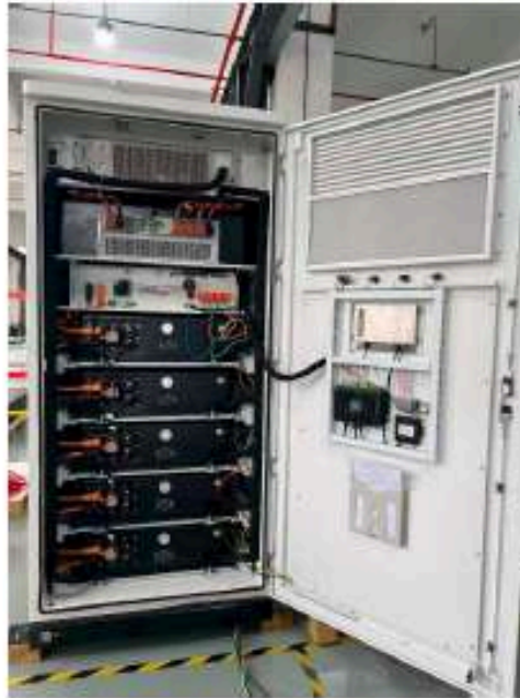
Energy Storage System (Open view)
