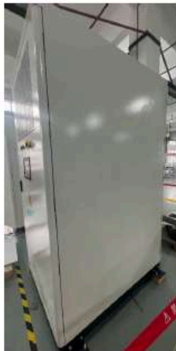
Energy Storage System (Right view)
