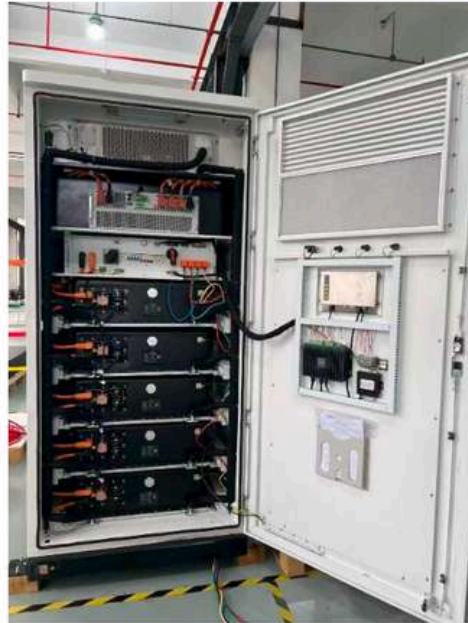
Energy Storage System (Open view)
