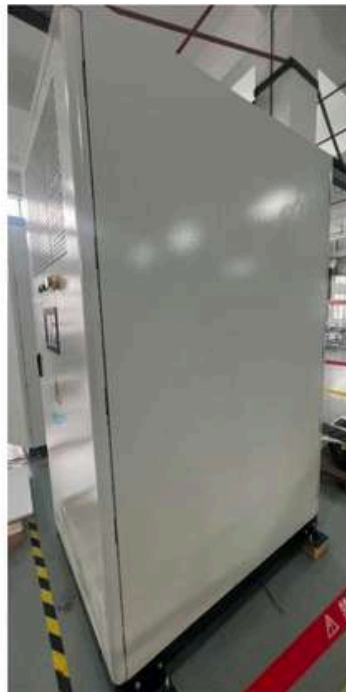
Energy Storage System (Right view)
