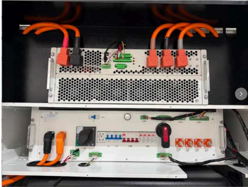
Battery control box
