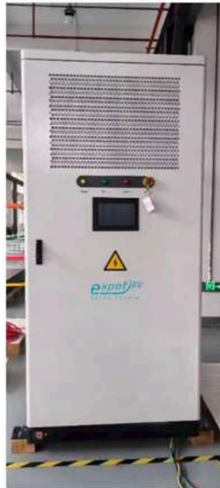
Energy Storage System (Front view)
