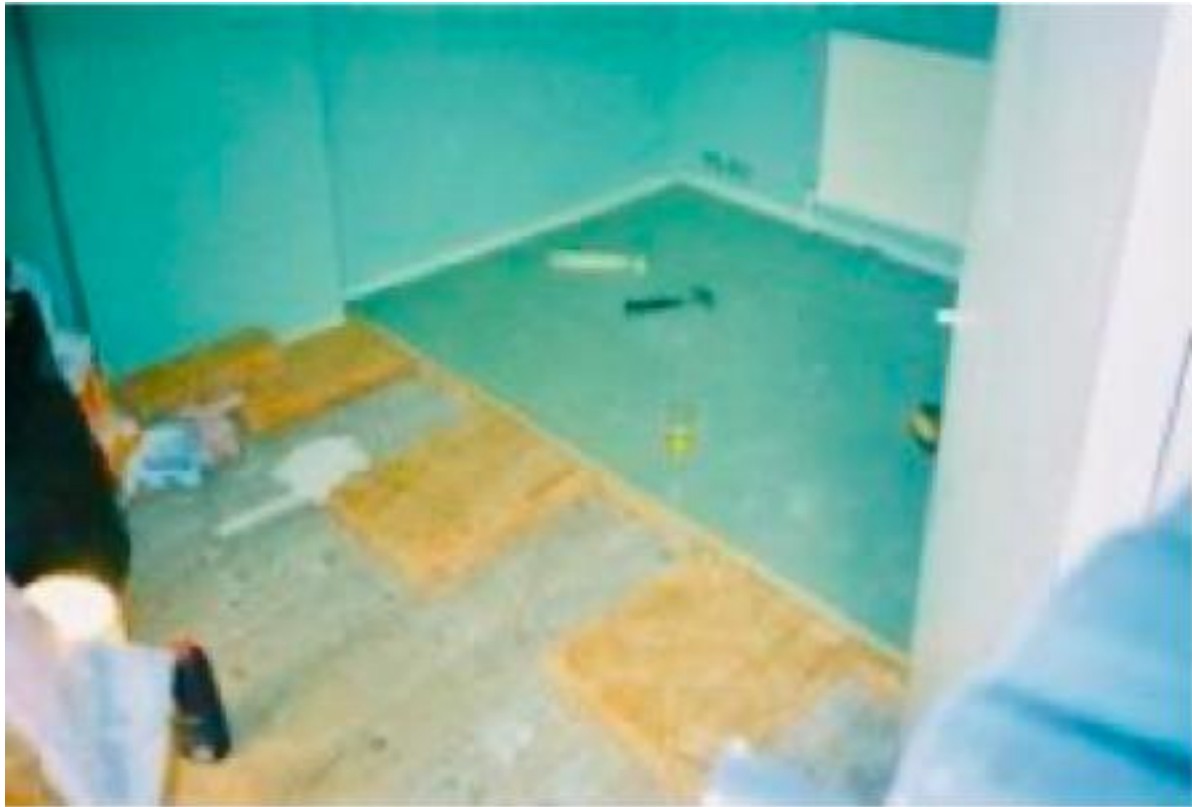
Photo - Floating floor. P5 chip wood floor laid on Rockwool - foam perimeter (C Daly 2022)
