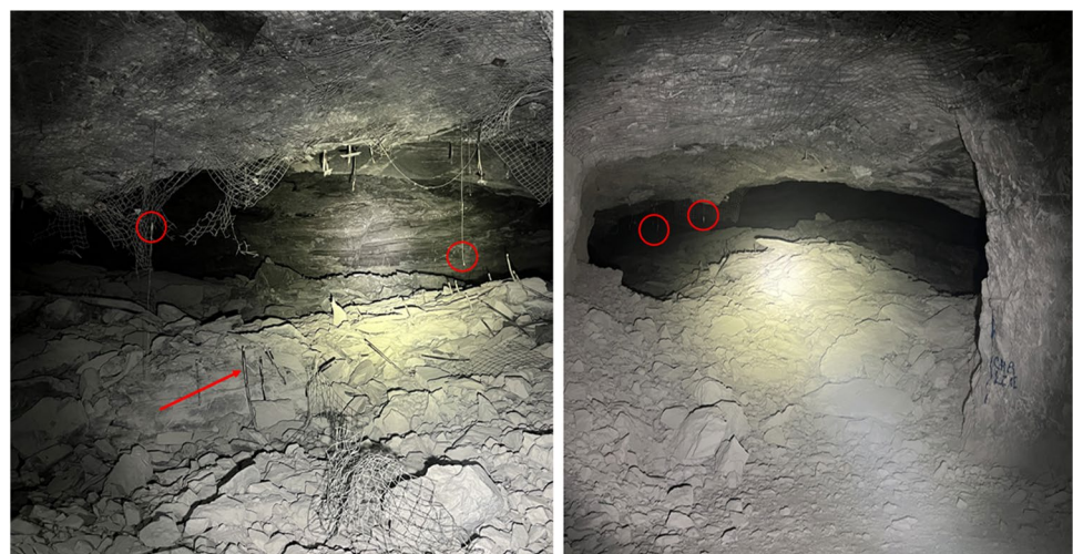
Fig. 8 Stope condition immediately after pillar removal. The red arrow indicates failed friction bolts noted in the stope. Red circles indicate locations where the fiber optic cable was severed between measurement boreholes
