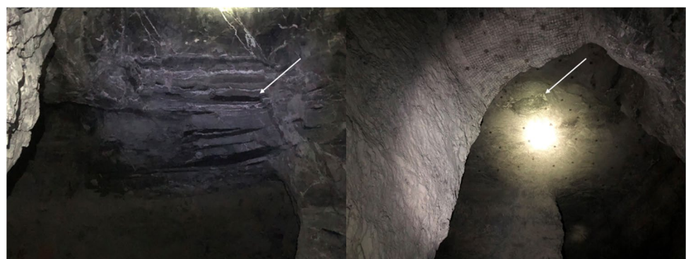
Fig. 4 (Left) Breakage to bedding planes noted in the measurement area. (Right) Small roof failure due to bedding separation in an area where the number 55 thin shale marker bed is in the immediate roof section
