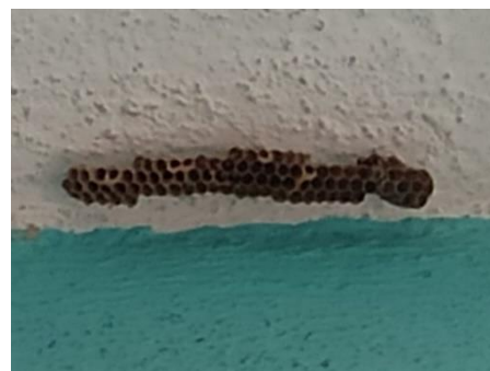
Fig. 2. Nest in the building ceiling
