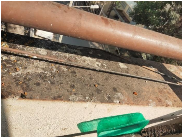
Sooty mold and dust on parapet wall
