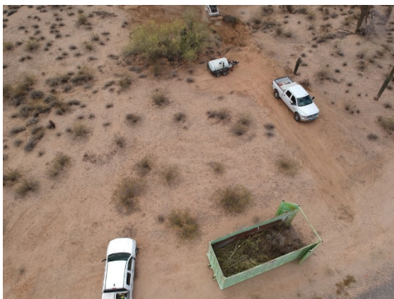
Beginning construction phase of the new Pyramid Peak, Simulcast G subsite for Peoria.
