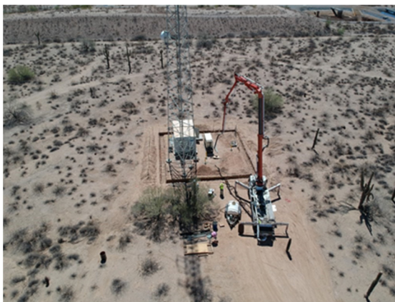
Construction of block walls at the new Pyramid Peak, Simulcast G subsite for Peoria.
