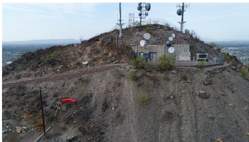
RWC communications site on North Mountain. This site is a primary hub for microwave connectivity.
