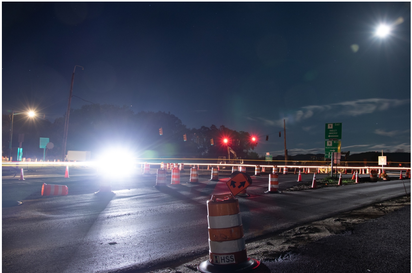
Figure 1: The new roundabout at I-91 Exit 19 / Route 9, Aug 4, 2020. Note the lack of artificial light, apart from vehicle headlights and one streetlight (at left), and the Full Moon (upper right). The current lighting plan would make the average illumination more than 200 times brighter than in this photo.
