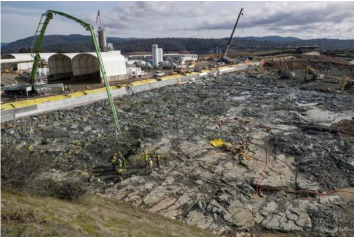
The repairs to the Oroville Dam spillway continue. It's an expensive fix to a poorly engineered dam.
