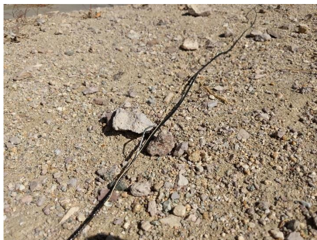
Figure 4 - Damage done to TD 2.0 counterpoise wire
