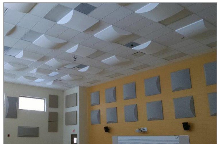
ESSI Barrel-Shaped Diffuser Panels inserted into existing hanging ceiling system and on walls
