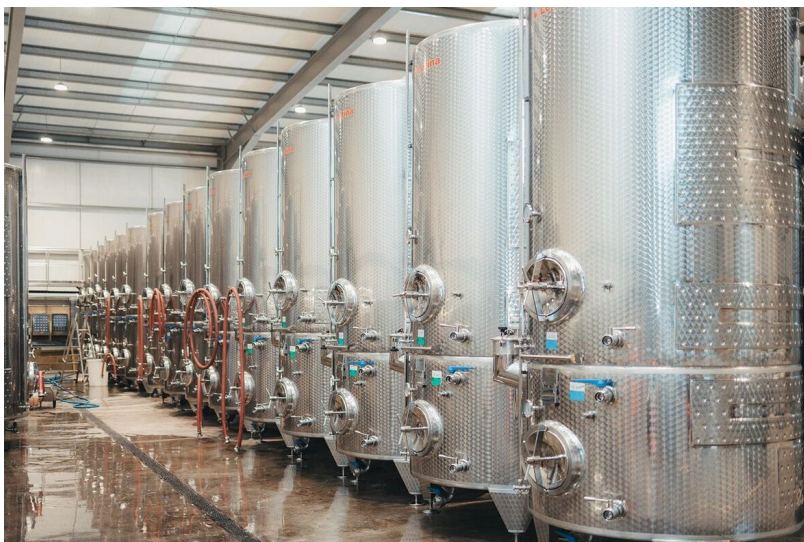
The East Anglia winery will have tanks like these (installed in Kent last year)
