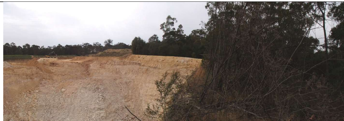
Plate 4: View of the working quarry pit with surveyed subject area on the right
