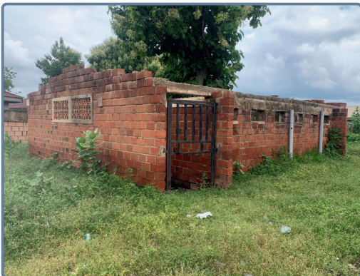
Before: An abandoned toilet facility at LEA Primary School, Phase 3, Gwagwalada
