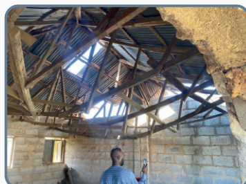
The state of the classroom before renovations at LEA Nomadic Primary School, Apo Dutse, Abuja.
