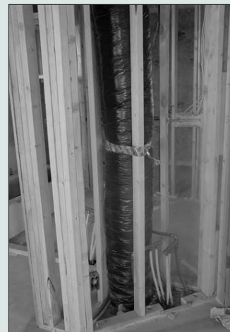
Courtesy of DOE/NREL. Credit: Warren Grete.
