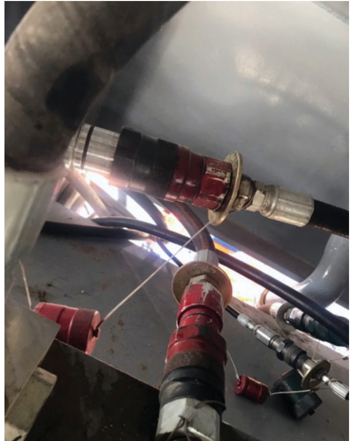
The cost of incorrectly connections (red connections pictured) can be costly in terms of NPT and safety risks
