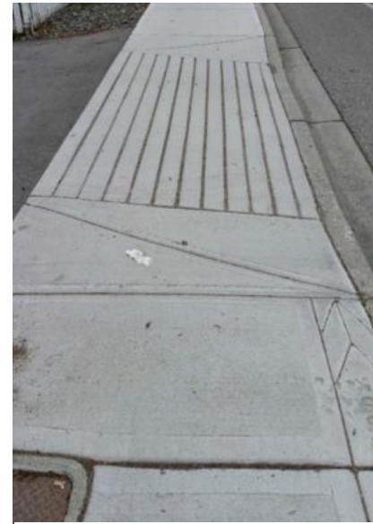
Figure 2 (above): A sidewalk after five years of use [4]
