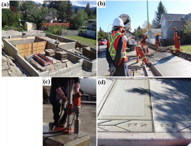
Figure 1(below): projects that use recycled concrete:(a) a casting of a foundation for a house (b) casting of a sidewalk (c) coring of a block (d) sidewalk with RCA content [4]
