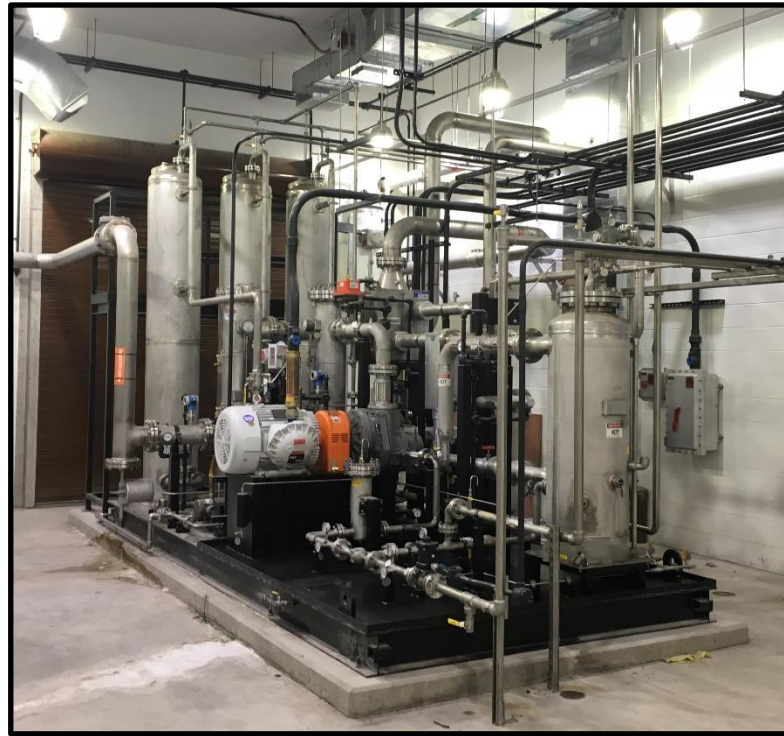
Gas Compression, Moisture, Siloxane/VOC Removal
