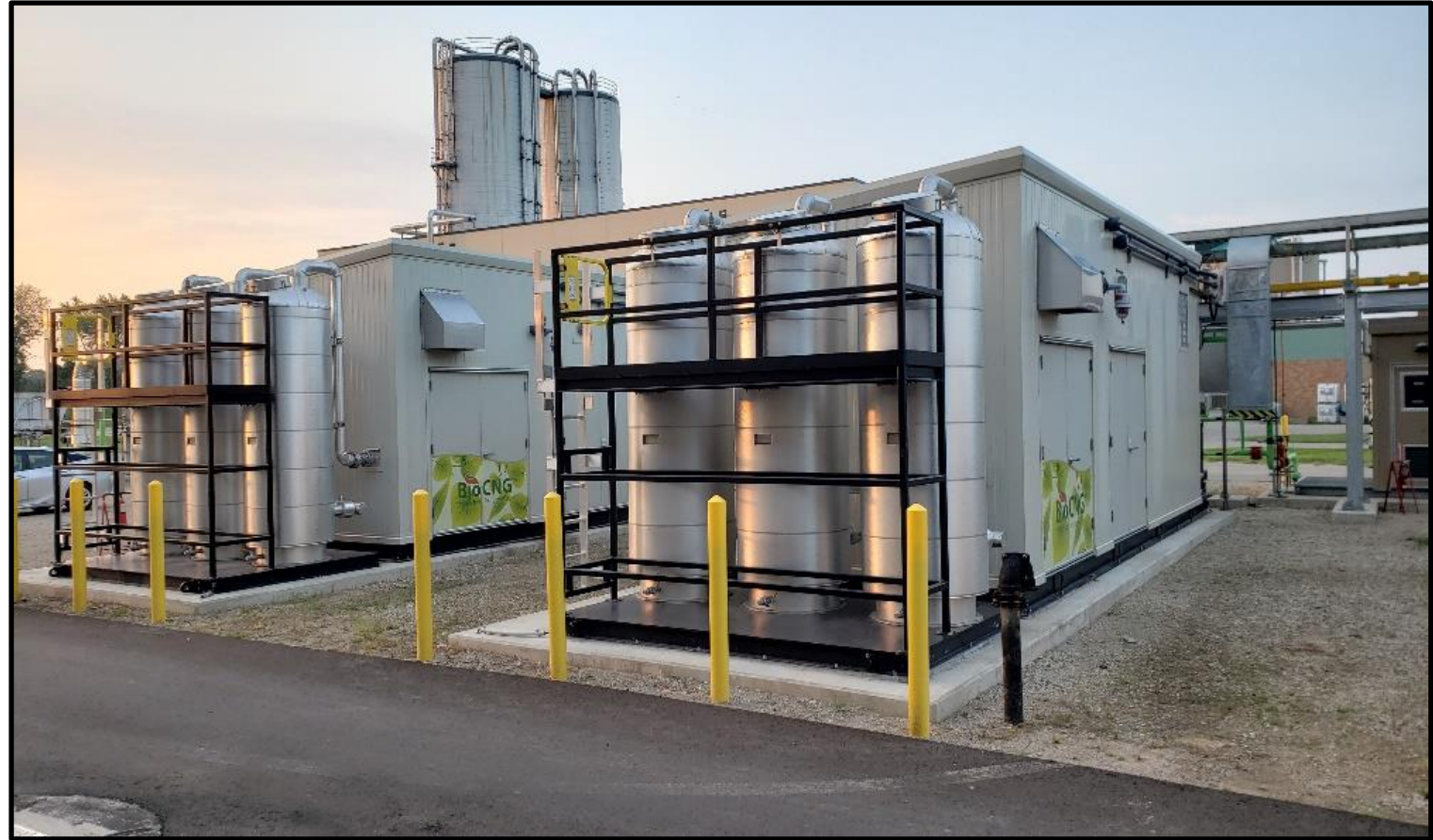
Gas Compression, Moisture, Bacteria, CO 2 and Siloxane Removal
