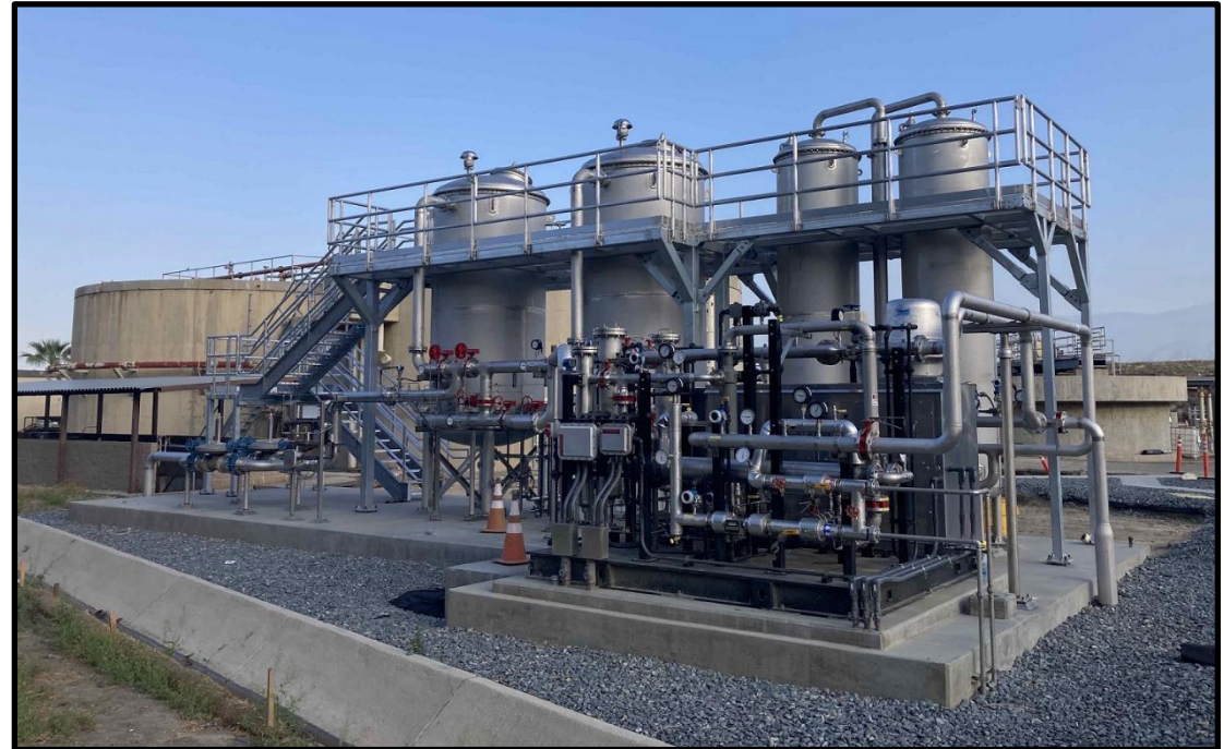
Gas Compression and Moisture Removal
