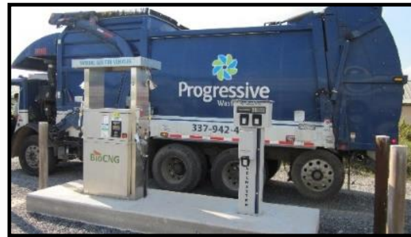
CNG Vehicle Fueling Station
