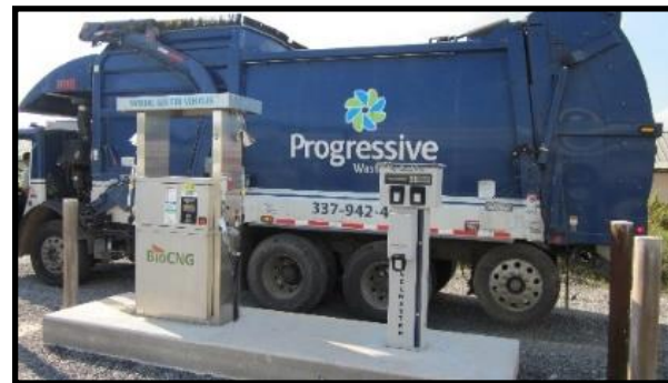
CNG Vehicle Fueling Station
