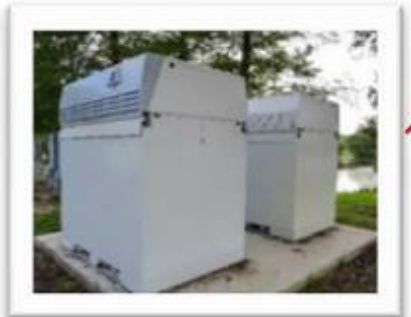
Two Vanadium Redox Flow Batteries
