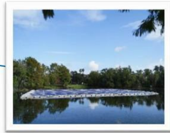
64kW Floating Solar Array
