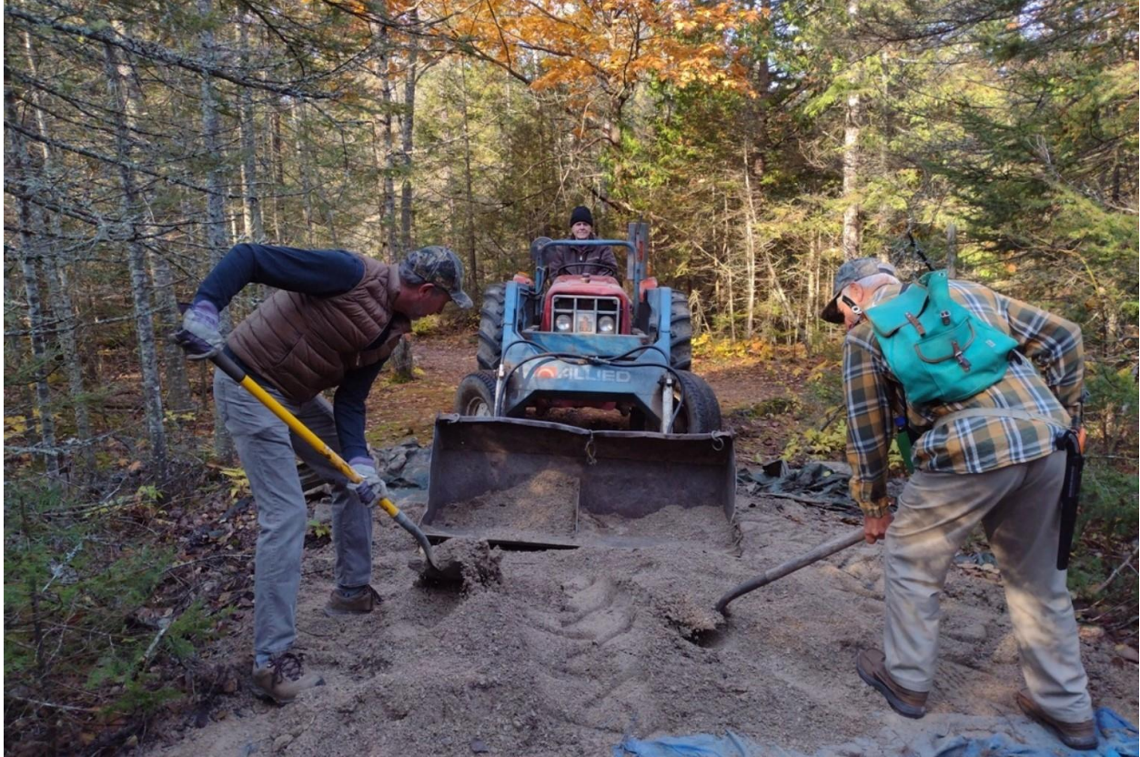
Left to right: Jim Cahill, Ron Bailey, David Kains moving the gravel pile (photo by Ken Mackenzie)
