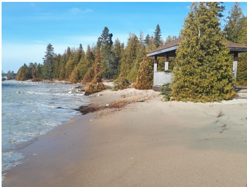
Picture of Shelter at Saunder’s Cove taken in mid fall. Lake levels had already started dropping by then. One can see where the storm wave surge swept partially under shelter. With the lake dropping- it should be okay for the winter season.
