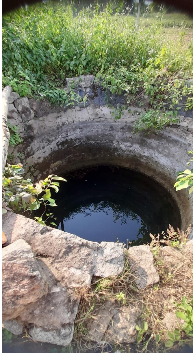
Picture: Unsafe Drinking Water used by PVTGs in Banaudha
