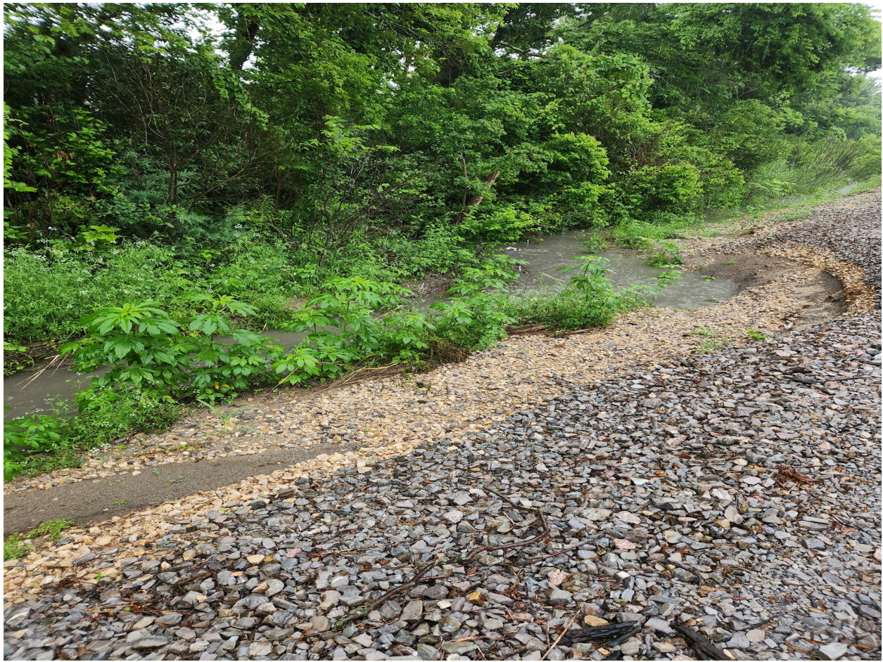
Erosion of the ditch bank and railroad base material.
