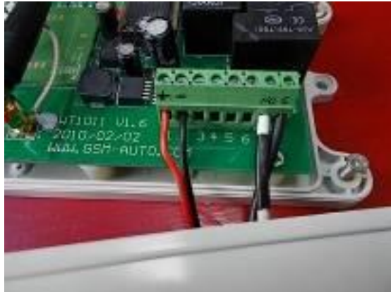
Figure 1: Wiring into terminals on Auto-GSM. The small red and black wires (terminal 1 and 2) come from the supplied transformer and provide 12VDC to power the circuits. The larger wires (terminal 8 "in" and terminal 7 "out") control the "hot" wire to the switched receptacles that power the engine heater.
