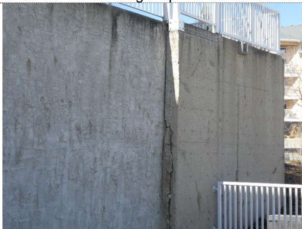
Damaged retaining wall
