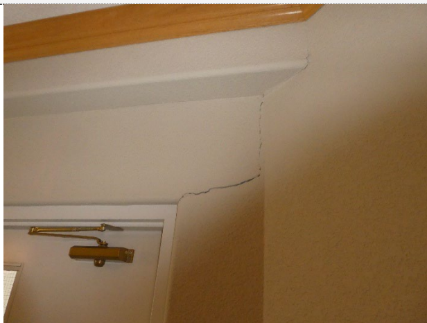
Settlement cracking (northwest corner)
