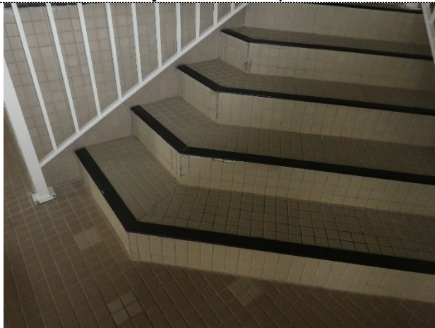
Minor damage to tile
