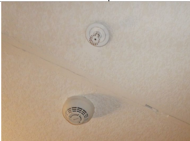
Sprinkler & smoke detector
