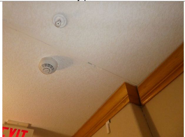
Cracking in ceiling
