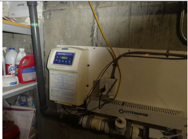
Pool Pilot – Chlorine generator
