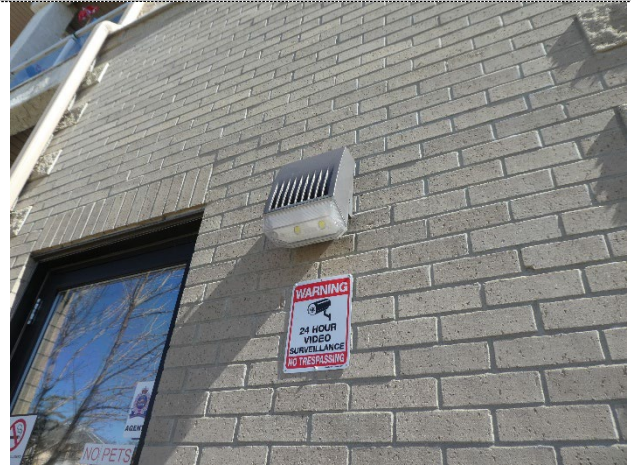
Exterior building lighting
