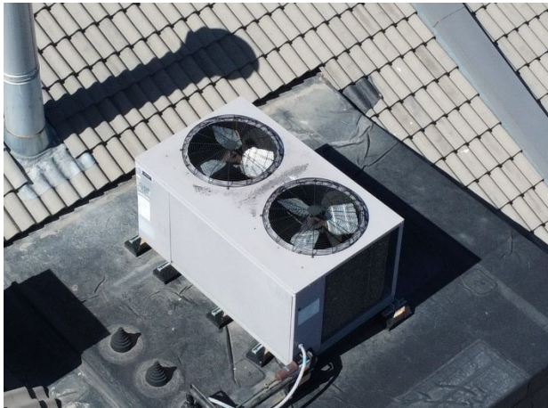
Rooftop A/C unit - Carrier M: 38AK5014 - 120 S: 4902F92298
