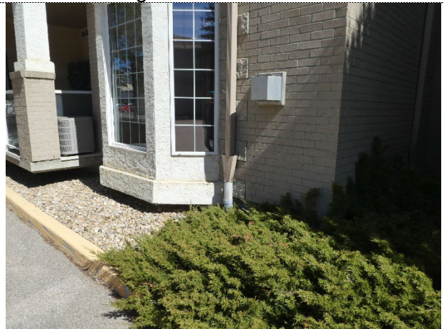
Downspout terminating into drain
