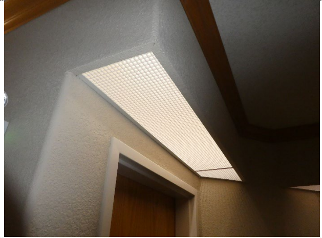
Interior lighting above unit doors
