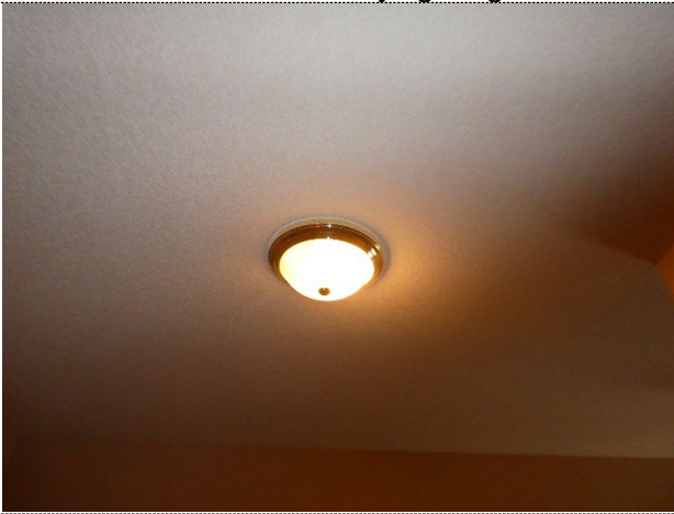
Miscellaneous incandescent lighting
