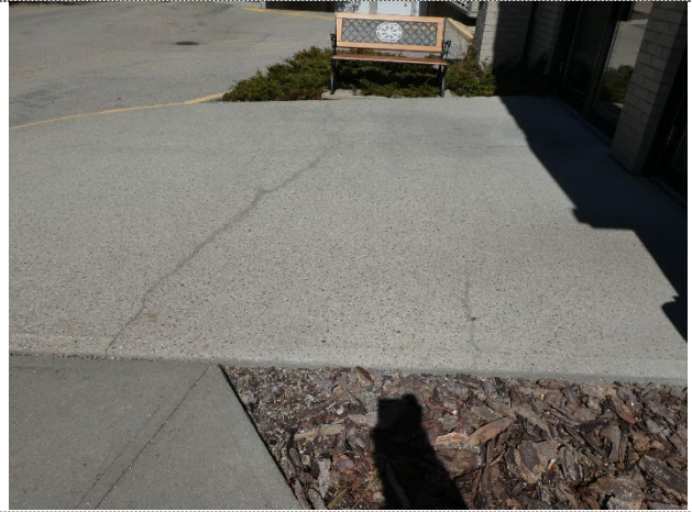
Cracking & spalling at entrance walkway
