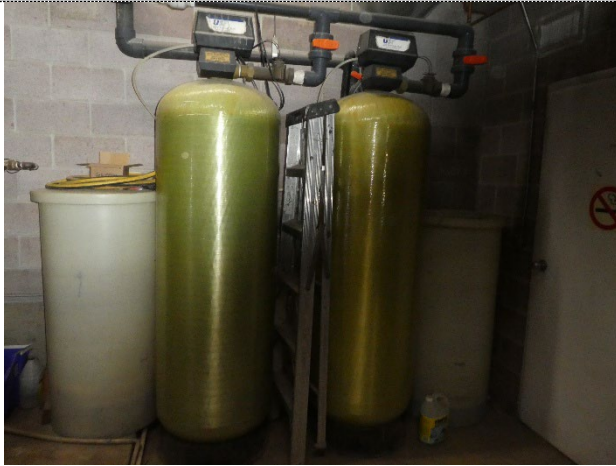
Water softener system
