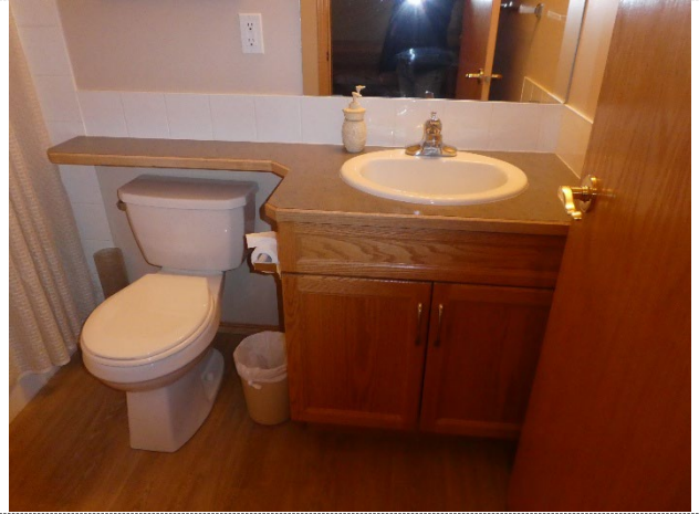
Guest room washroom fixtures
