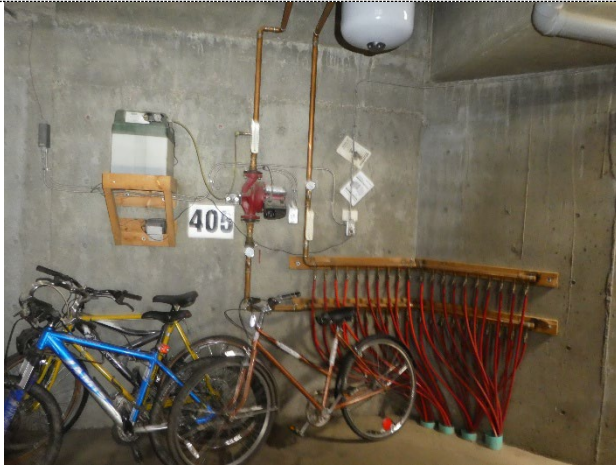
Glycol heat loop mechanical components
