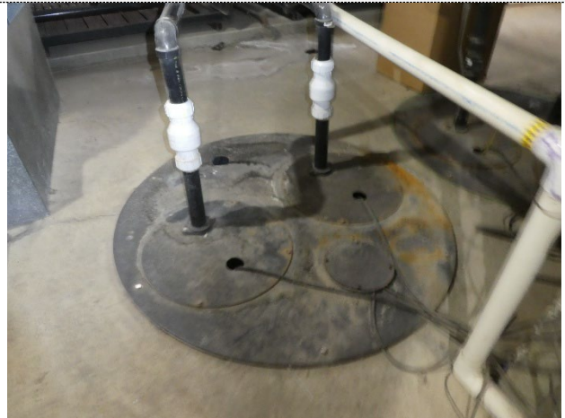
Sump pump location
