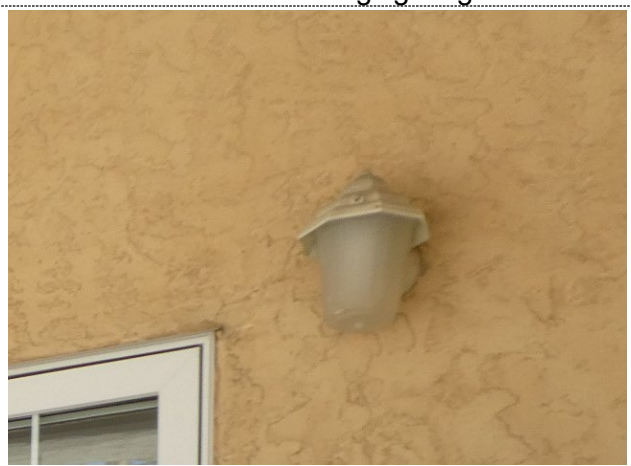
Typical unit lighting
