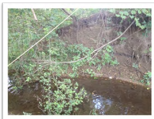
Photograph 3 (8-26-12). Excessive streambank erosion is widespread with large amounts of bare soil.
