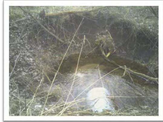
Photograph 2 (02-02-12). Water emerging from a culvert beneath CR 550 South is eroding the ditch bank.
