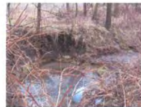
Oliver Lake-10 Facing SW from 550 S. at erosion on...
