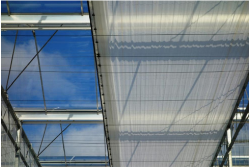
Retractable shade nets can be deployed inside a greenhouse to reduce light intensity.
