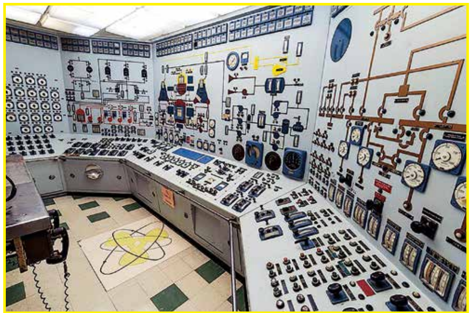
The engineering control room aboard the NS Savannah .
