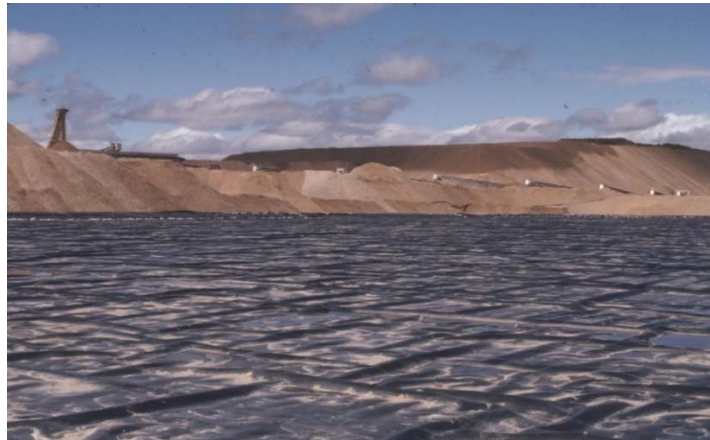
Fig. 4. Example of geomembrane wrinkles in two perpendicular directions [Photo J.P. Giroud].
