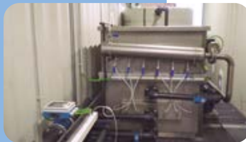
DAF in container
