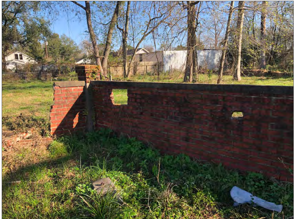
Figure 25. Damage to the Westcott brick wall, including the toppled arch (McDoux)
