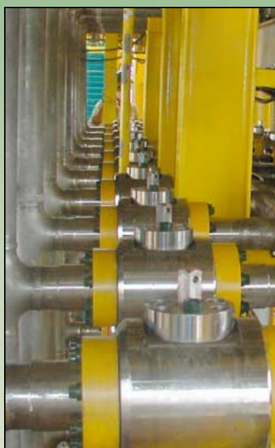
Manifold assembly prepared for actuator installation.
