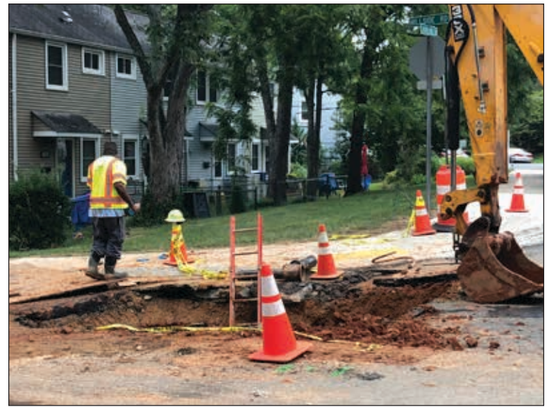
A big hole and warning cones mark the water main break at Hillside and Laurel Hill Roads.
