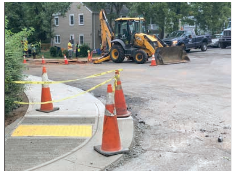
Newly minted sidewalks are ready for the new road surface across from the water main break at Hillside and Laurel Hill.
